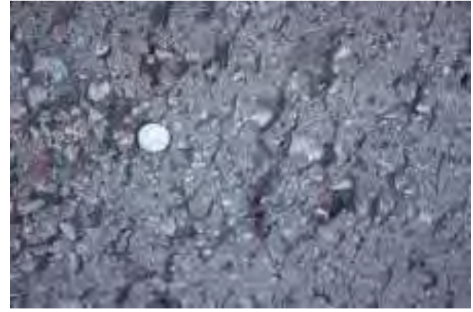
Sludge Drying Bed, TX
